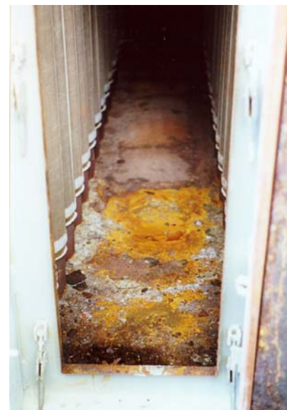
Figure 6 – Tube Sheet Corrosion
