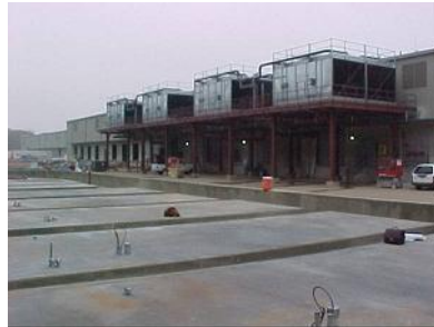
Figure 2: Direct Cooling Towers on an Elevated Platform
