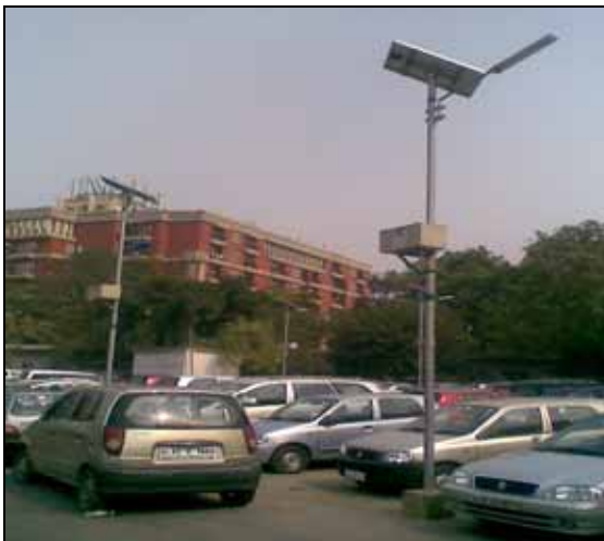
Solar Lights in Station Parking areas
