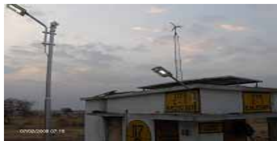
Hybrid (wind mill + Solar) LED lighting at LC gate
