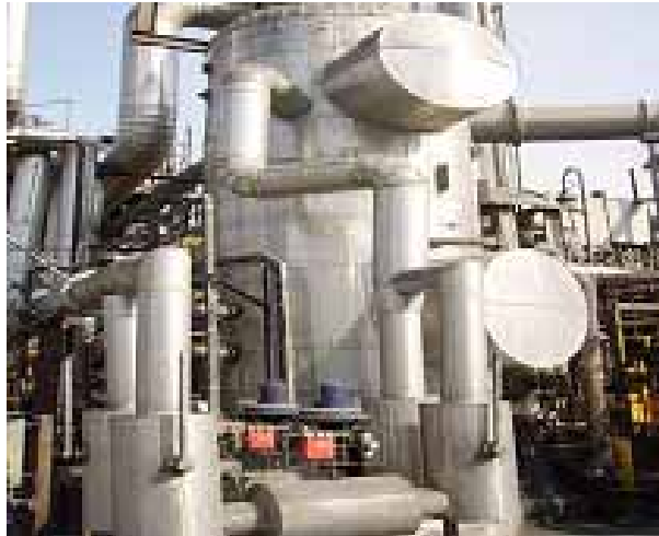
Ammonia Wash Unit
