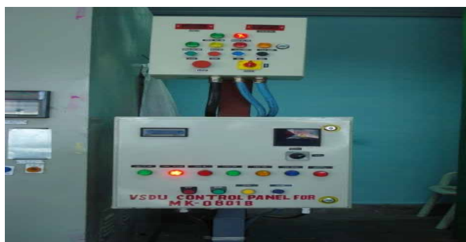
Variable Speed Drives Panel
