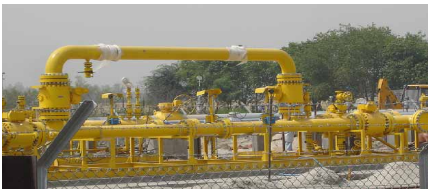
GAIL Terminal at Phulpur Unit
