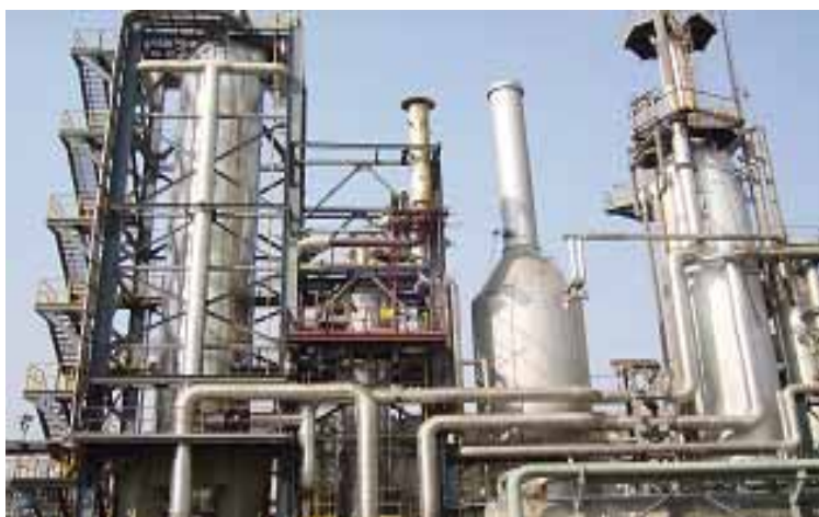
S-50 Converter and MP Boiler
