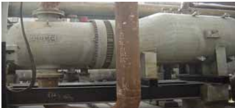
Final Gas Chiller
