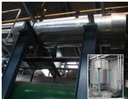
New De- Super Heater For Chilled Water Plant & Hot Water Collection Tank with Pump (Inside)
