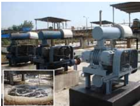
New Defused Aeration System Blowers & Aeration Tank (Inside)
