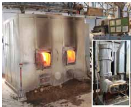
Modified Briquettes Fired MR-12046 Boiler With Economizer and Blower (Inside)
