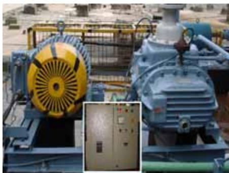
New PCN Mechanical Booster With VFD Control Panel (Inside)
