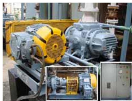
EDC Mechanical Booster With New (Inside) HE Pump CPKE-50/160 With 10HP/2900 RPM EFF1 Motor & VFD Panel For Mechanical Booster
