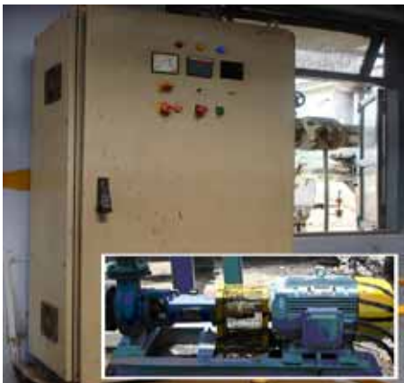
New VFD Panel For Chilled Water Primary Pumps ( Inside Mega-G-80/160 Pump with EFF1 50 HP Motor)
