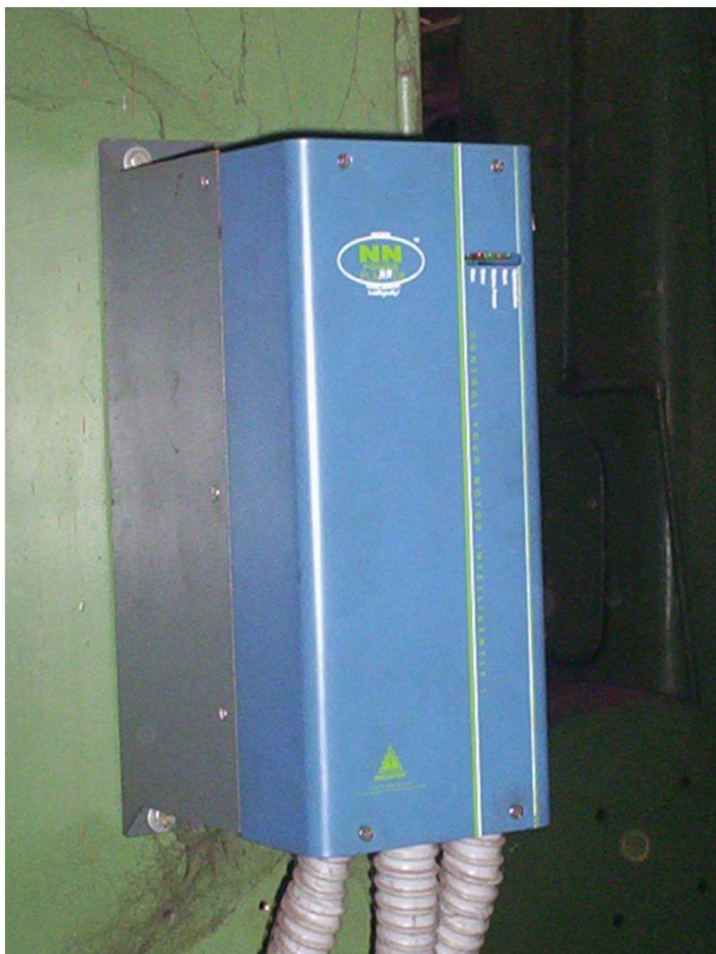
Energy Saver at Electrical Machines in Mechanical Workshop Gorakhpur
