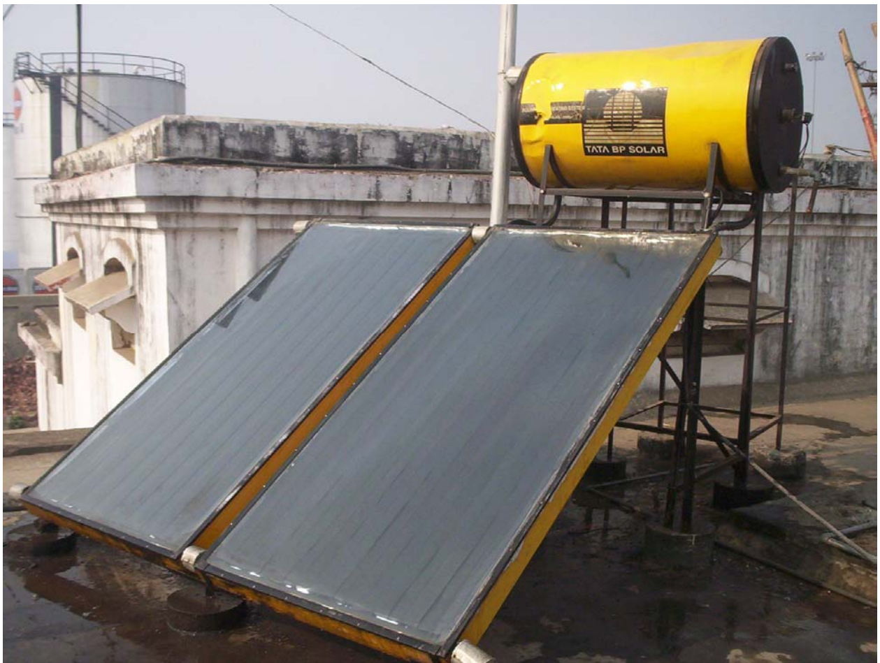
Solar Water Heater at Running Room Gorakhpur
