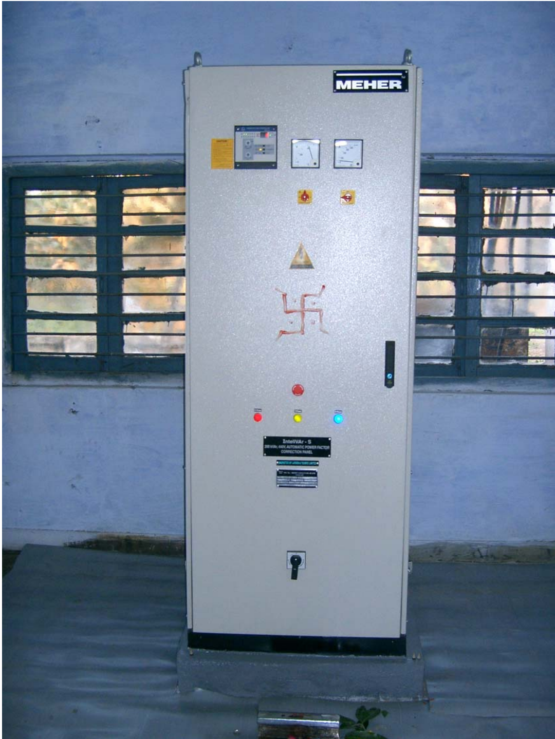
200 KVAR APFC Panel at DRM Office Izzatnagar
