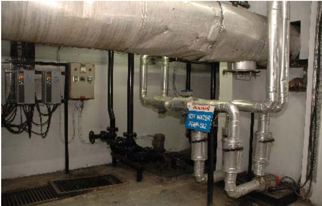
HOT WATER PUMPING FROM DESUPERHEATER TO CALORIFIER
