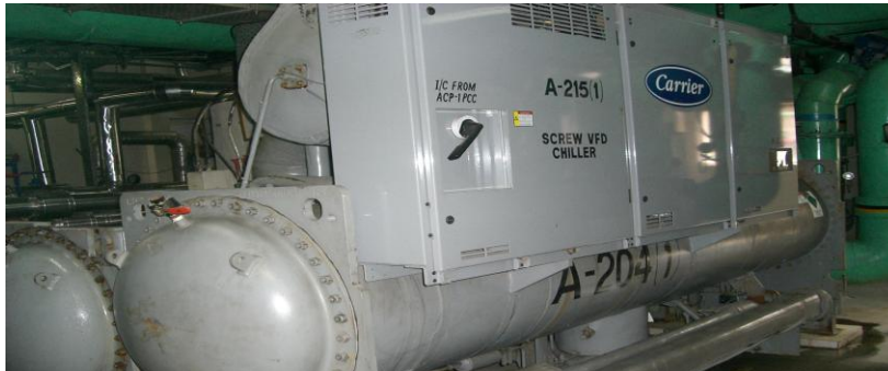
Energy Efficient VFD Screw Chillers (02 Nos)
