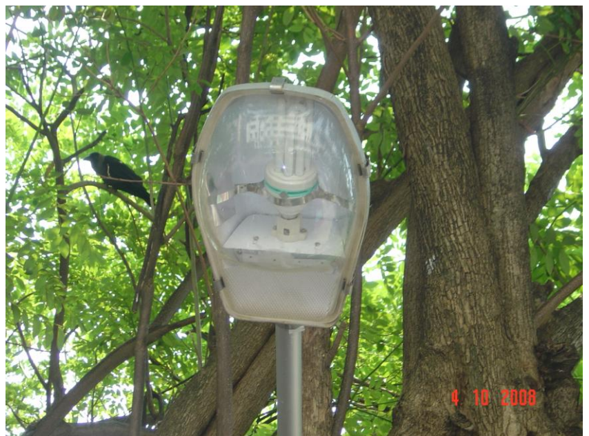
CFL street light
