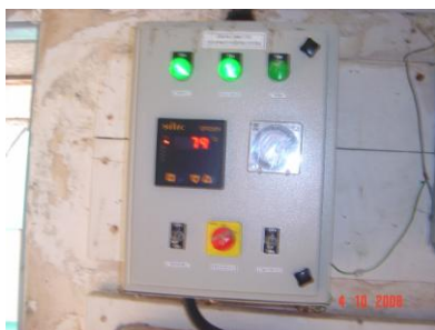
Control panel for above system
