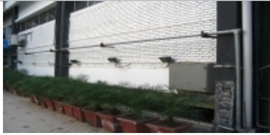
Soap free water pipeline going to the garden
