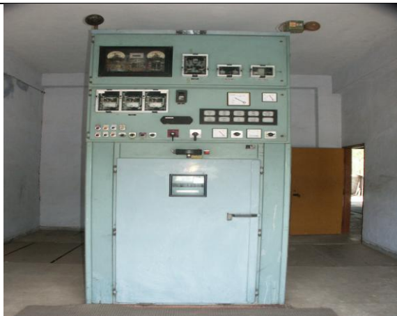
22 KV H.T. Panel (MOCB)
