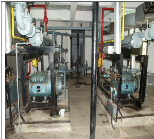
2 x 30 TR Reciprocating Compressors
