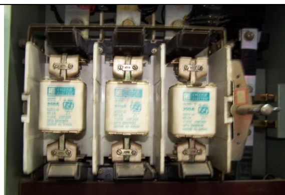
Feeders with HRC Fuses (SFU) –Existing
