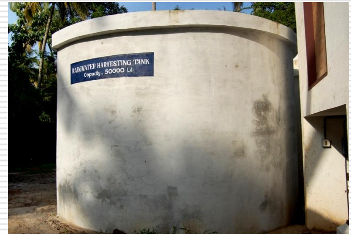
Rain harvesting tank.
