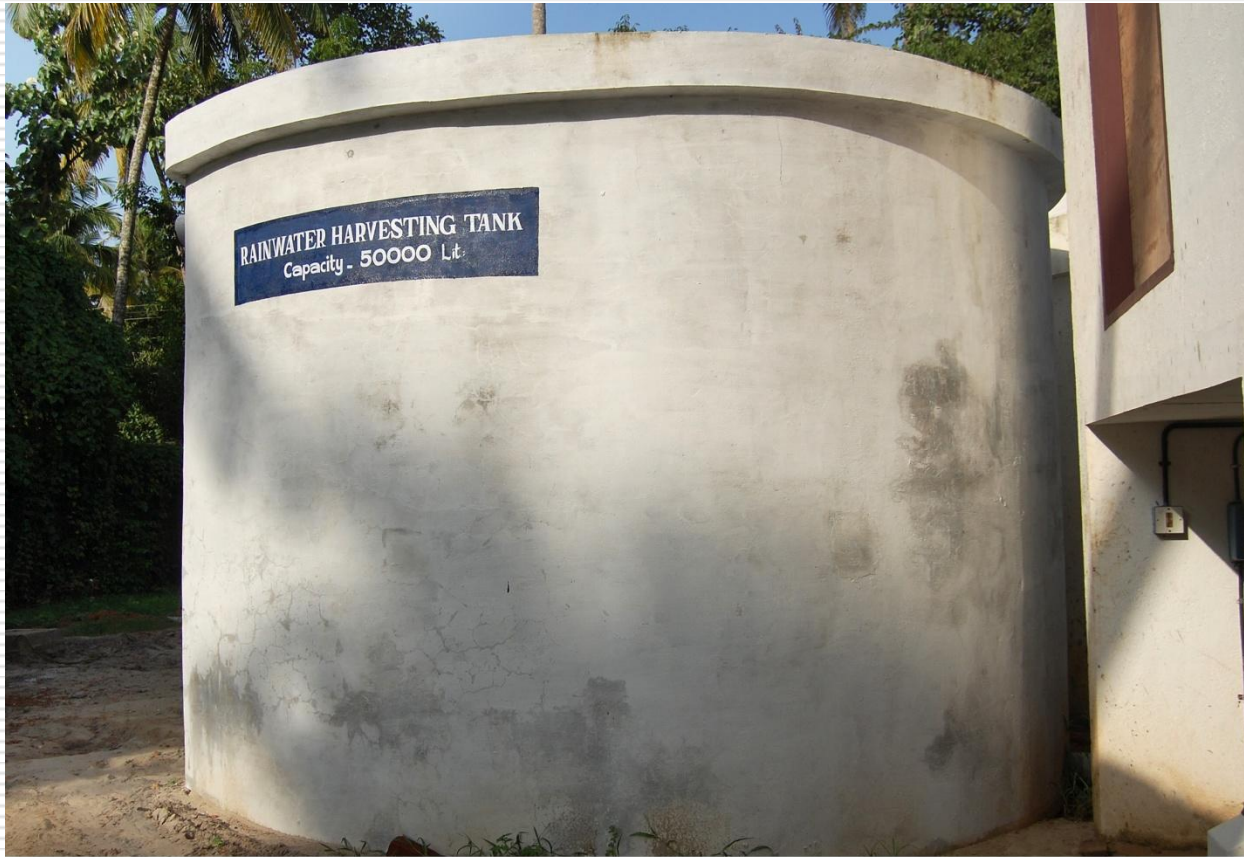
Rain harvesting tank.
