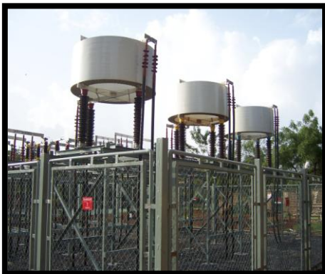
3 phase Series Reactors
