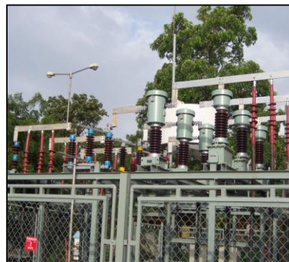
Mini switch-yard for HVSR
