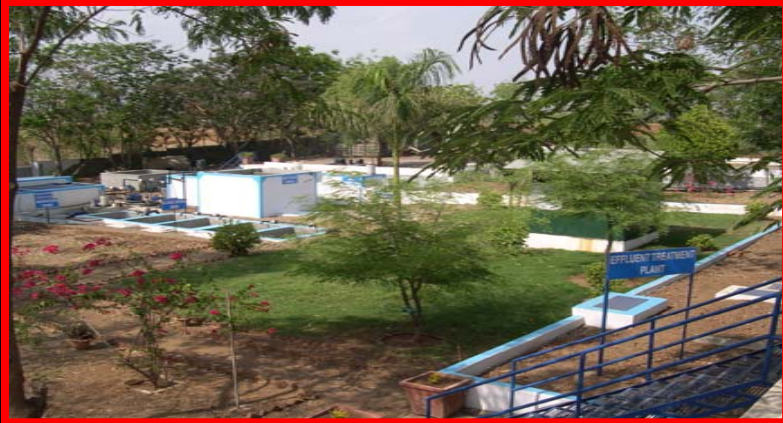
Effluent Treatment Plant
