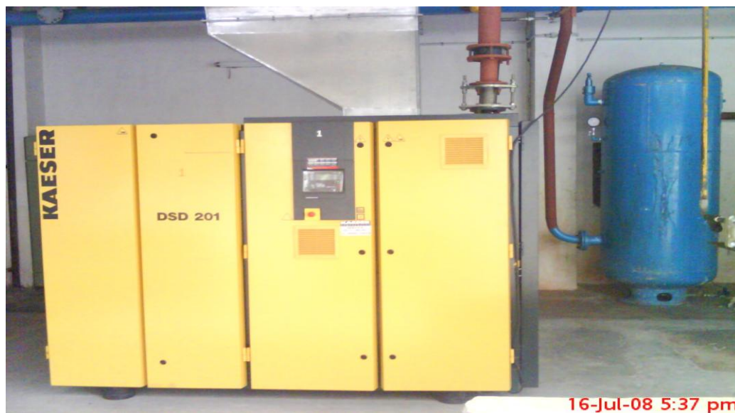
OVER VIEW OF KAESER MAKE DSD 201 COMPRESSOR
