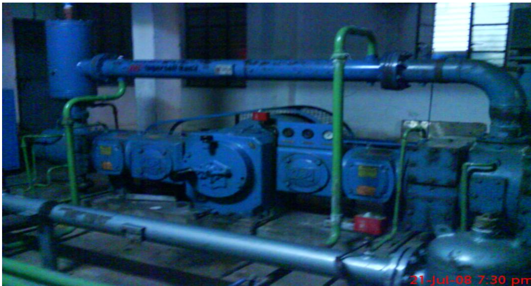
VIEW OF I.R. MAKE IHE – 5 COMPRESSOR
