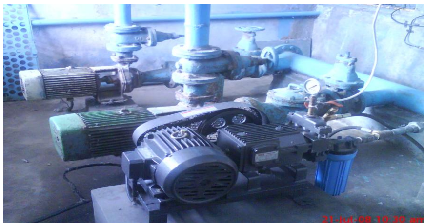
OVER VIEW OF PUMPS
