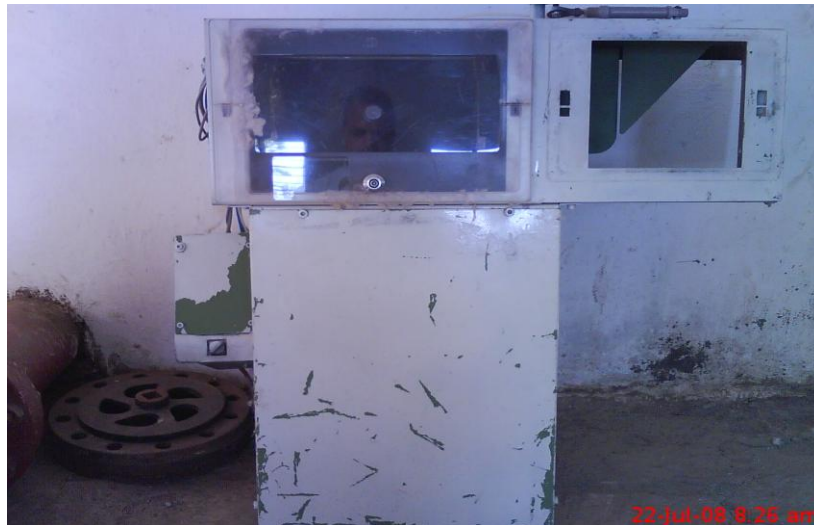
OVER VIEW OF DUST SUCTION FAN
