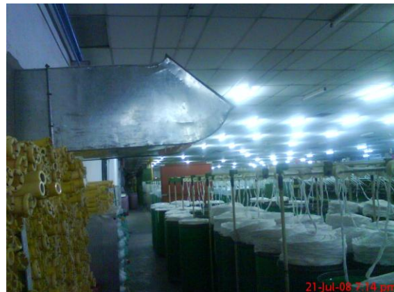
HOT EXHAUST AIR OF COMPRESOR
