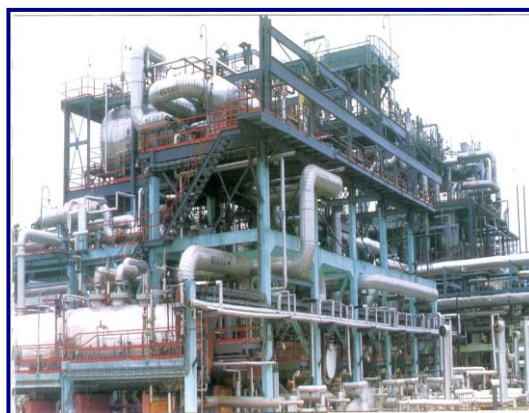
Sulphur Recovery Unit
