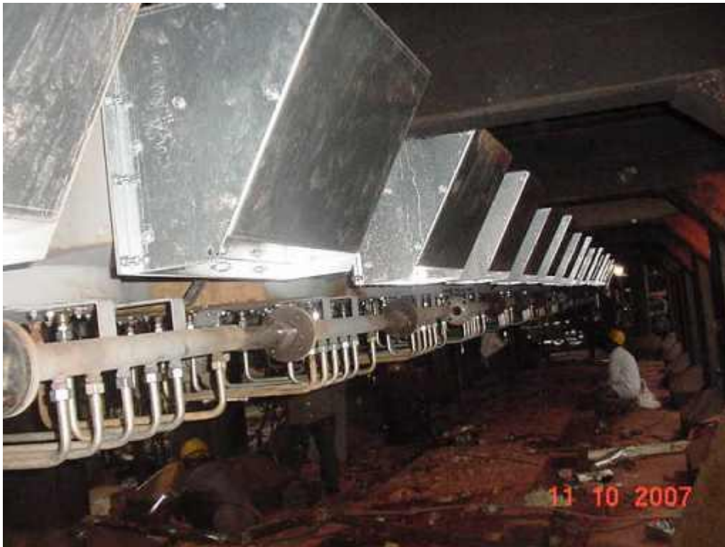
New Low Excess Air Burners installed in VBU
