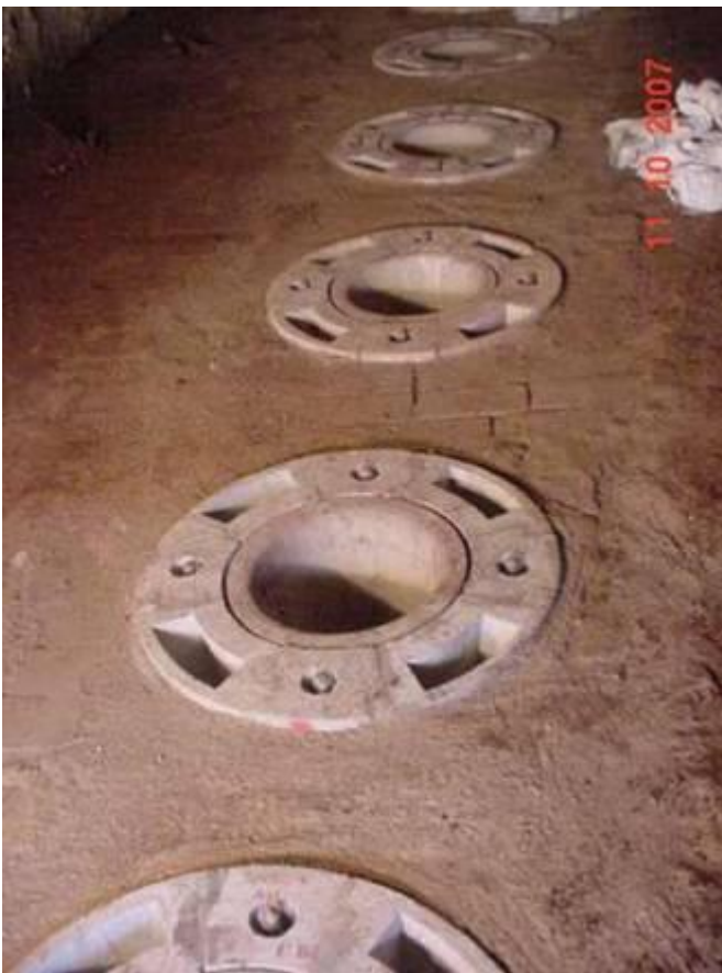
New Low Excess Air Burners installed in PDA
