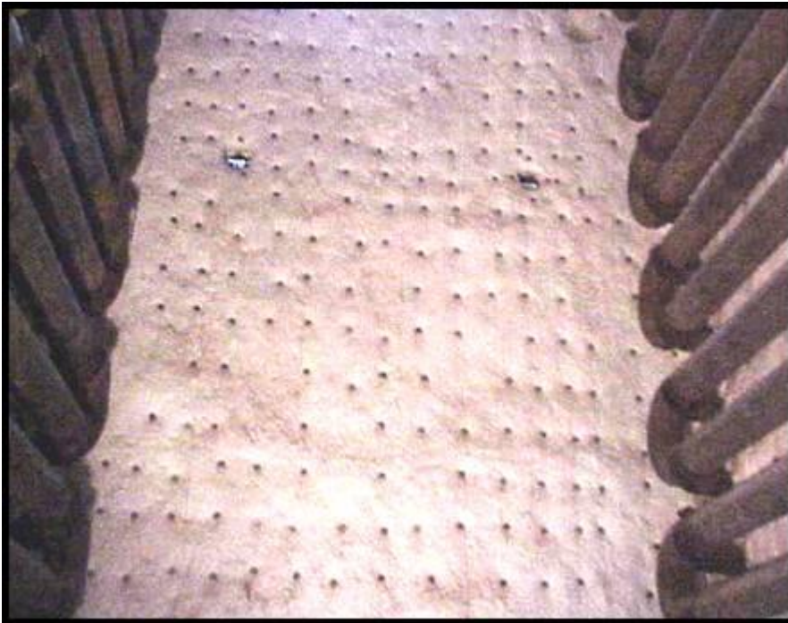
Ceramic Insulation inside PDA Furnace
