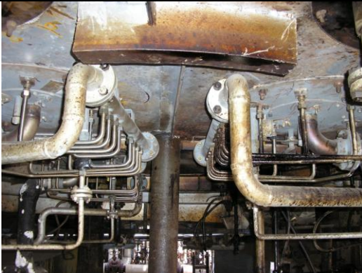
Bottom view of off gas burners installed
