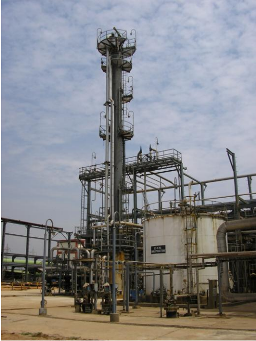
View of the new plant
