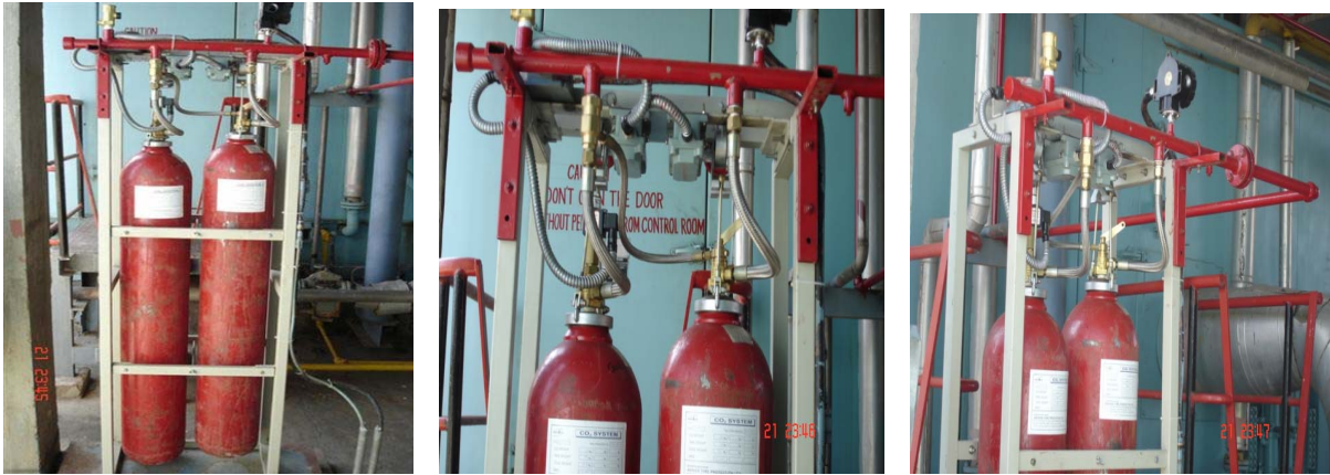
HALON REPLACEMENT WITH CO 2
