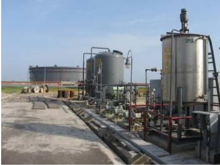
ETP in Shore tank farm
