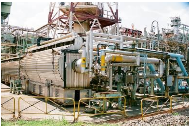
Reduction Furnace in DHDS SRU unit.
