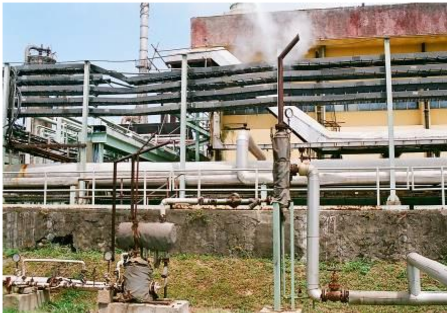
Condensate Recovery System at Plant Fuel tank farm
