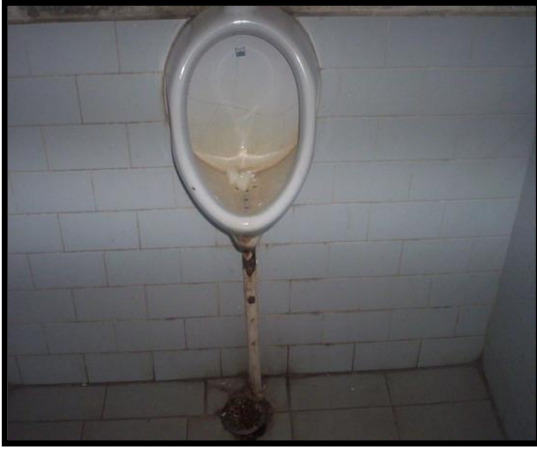
BEFORE (WATER FLUSH URINAL)
