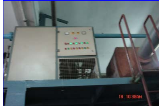
Brine system of 5 TR capacity, Chikhalthana Plant
