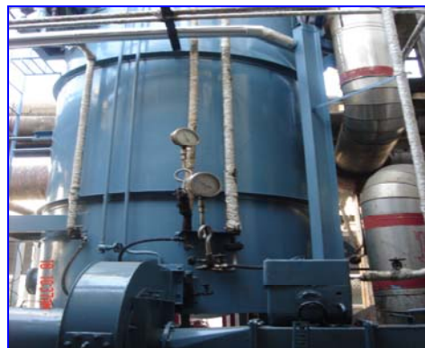
Thermic Fluid Heater – TP 15, Chikhalthana Plant
