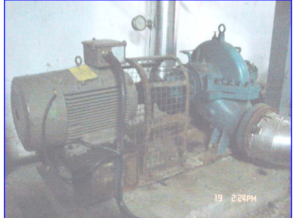
New High efficiency pump, Chikhalthana Plant
