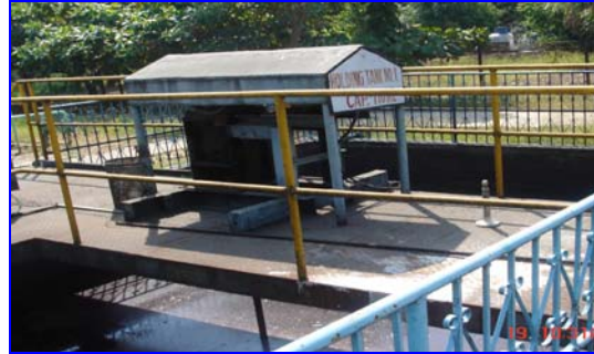
Chikhalthana Plant ETP incoming effluent tank agitator.
