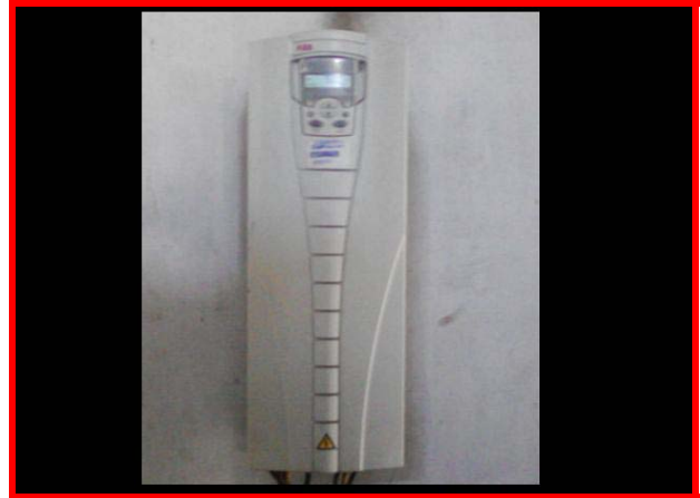
VFD for VAHP cooling tower
