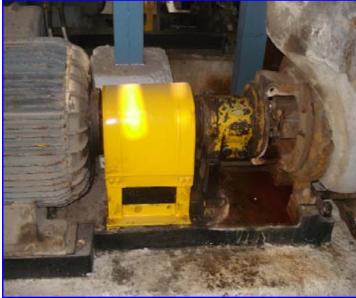
Old inefficient pump, Chikhalthana Plant
