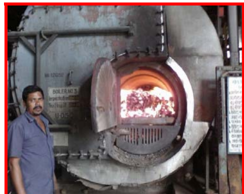
Bio-Coal fired Boiler
