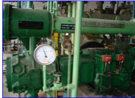
2 Nos. of LT reciprocating compressor of lower capacity 600NM3/Hr. were installed
