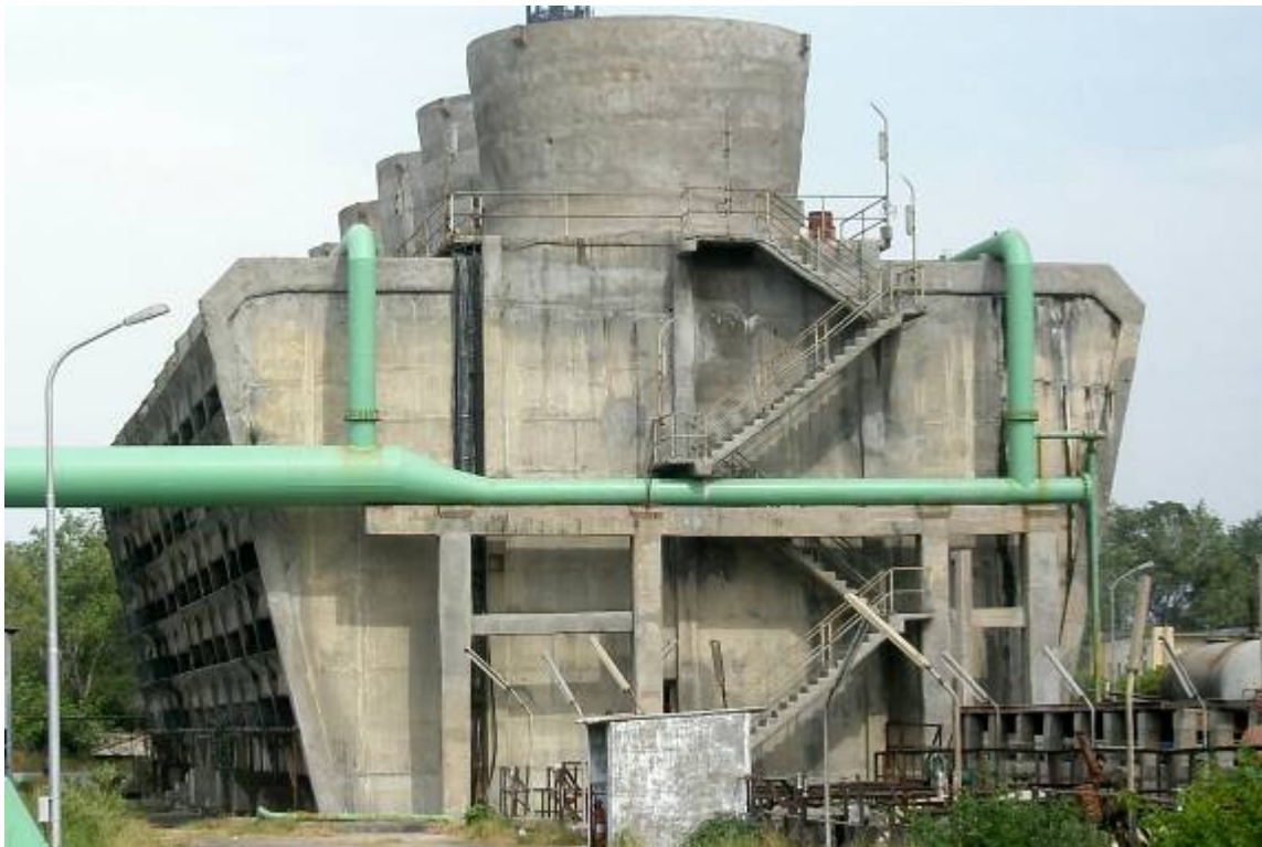
( Photograph showing Cooling Tower of Utilities plant where energy efficient pump was installed in place of less efficient one.)
