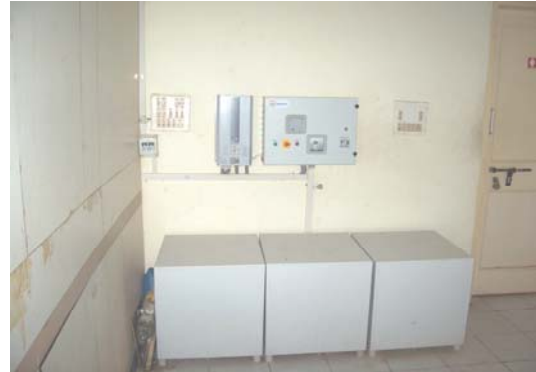
Solar Light Battery Bank
