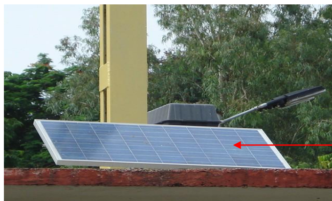
Solar lighting system
