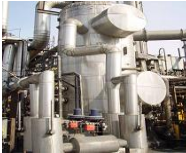
Ammonia Wash Unit
