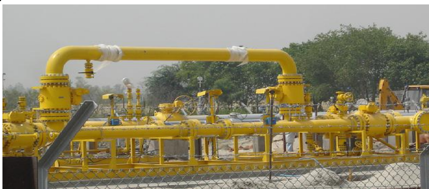
GAIL Terminal at Phulpur Unit
