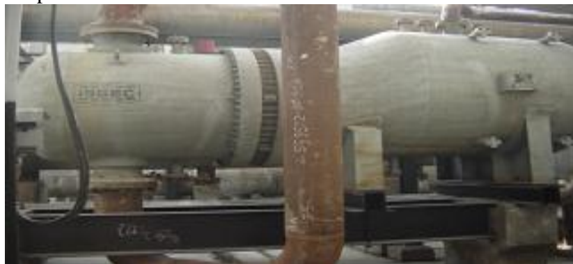
Final Gas Chiller
