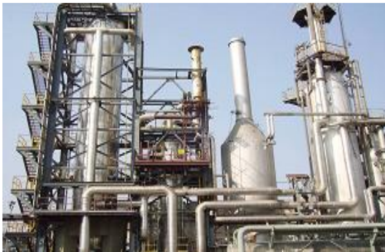
S-50 Converter and MP Boiler
