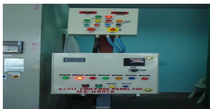
Variable Speed Drives Panel
