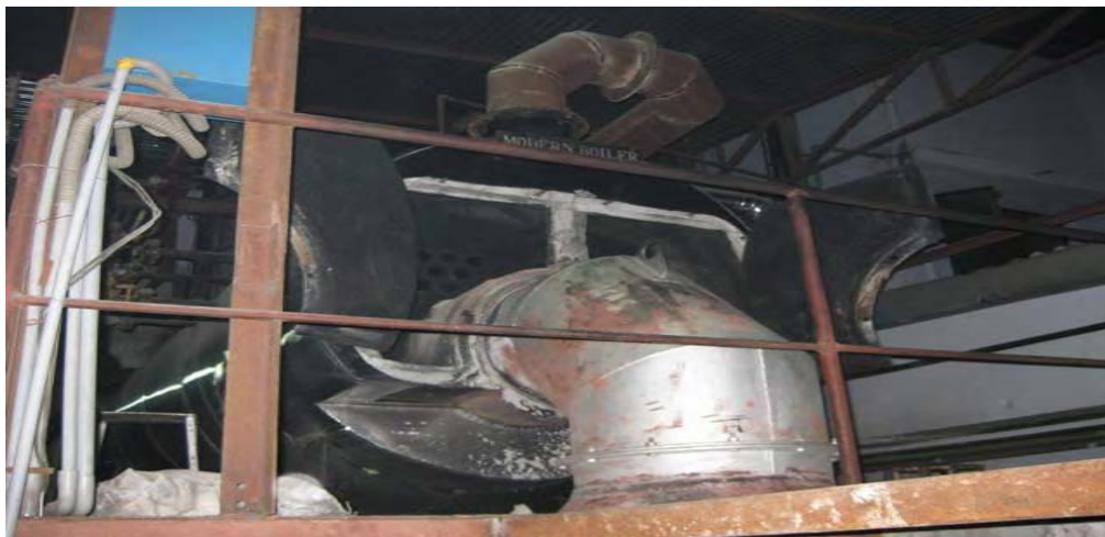
Front Open Portion of Briquettes Boiler – 1.2 Ton
