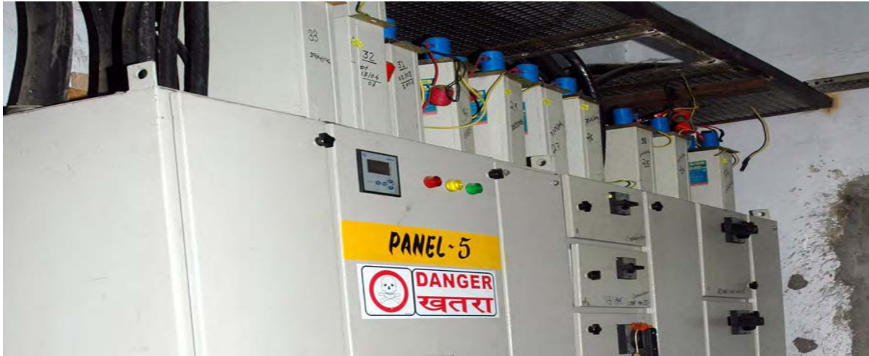
CAPACITOR BANK No. 1
