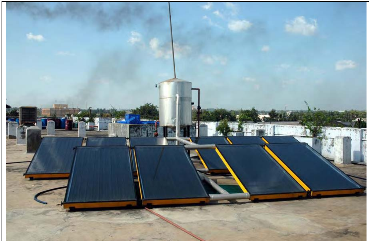
Solar Energy Utilization system by Solar Heater
