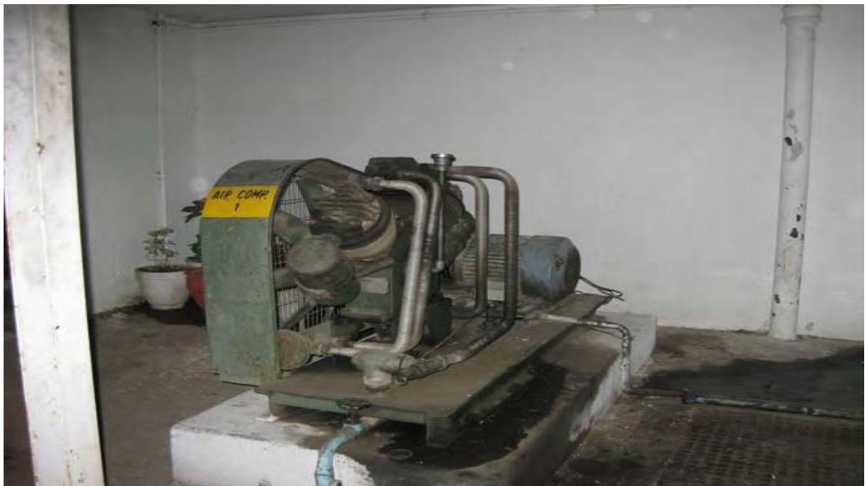
Elgi Make Air Compressor
