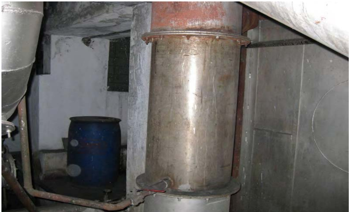
SS Economizer attached between IBR Boiler and Chimney
