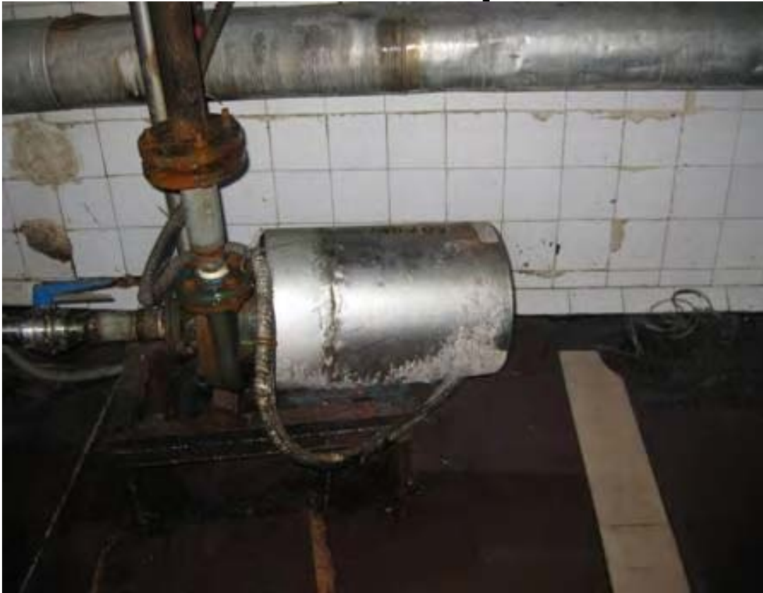
3 Hp Chilled Water Pump
