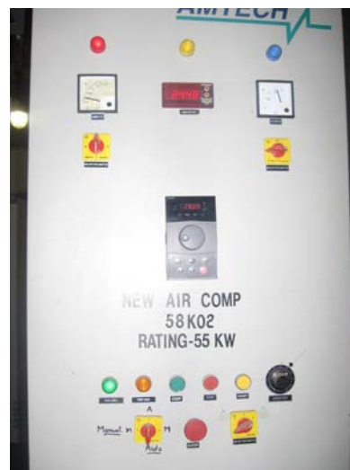
Air Compressor VFD
