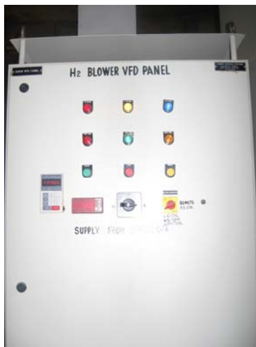
H2 Blower VFD
