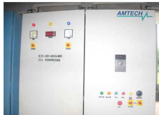
Chlorine compressor VFD
