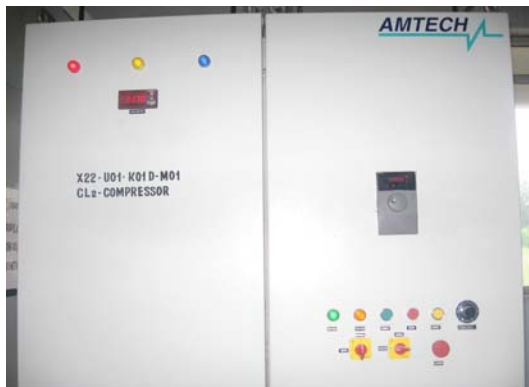
Chlorine compressor VFD
