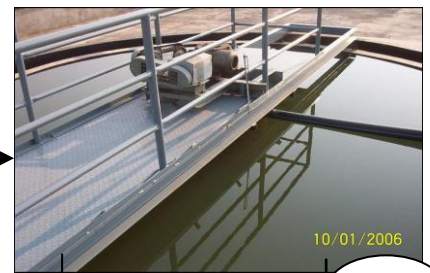
Top view of clarifier
