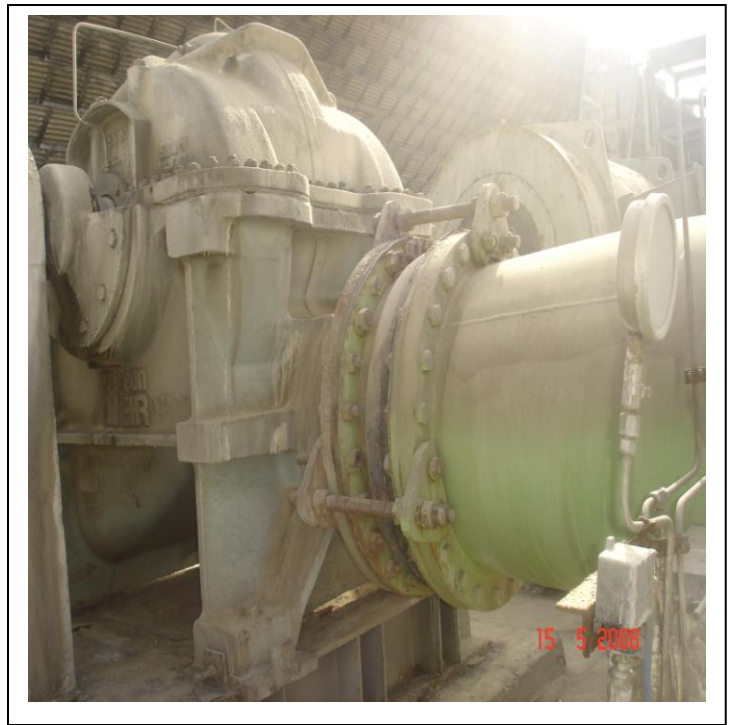
Coro-coating of Ammonia cooling water pump to save electric power
