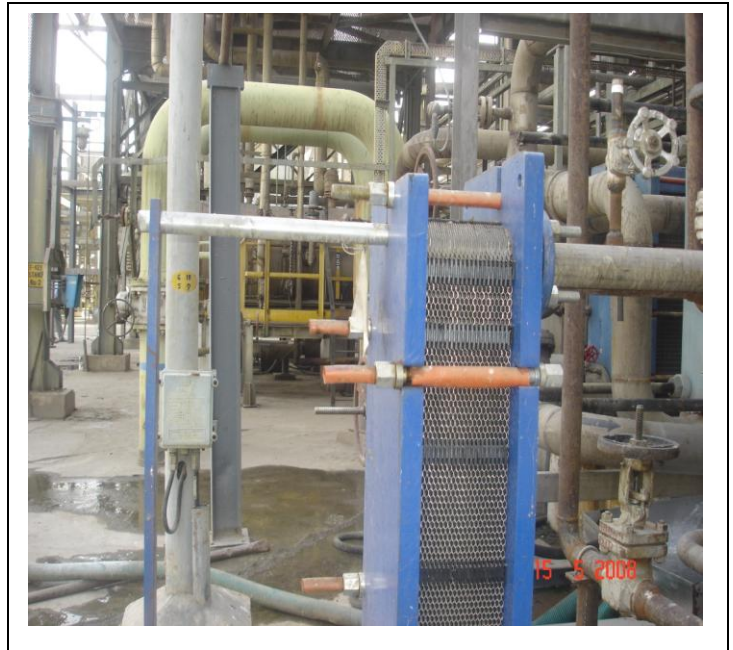
Installation of Plate type heat exchanger to recover Boiler blow down heat
