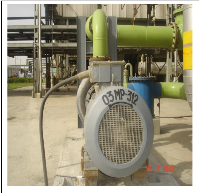
Installation of Booster pump for Syn gas final cooler (E-312) in ammonia plant vessels (ME-
