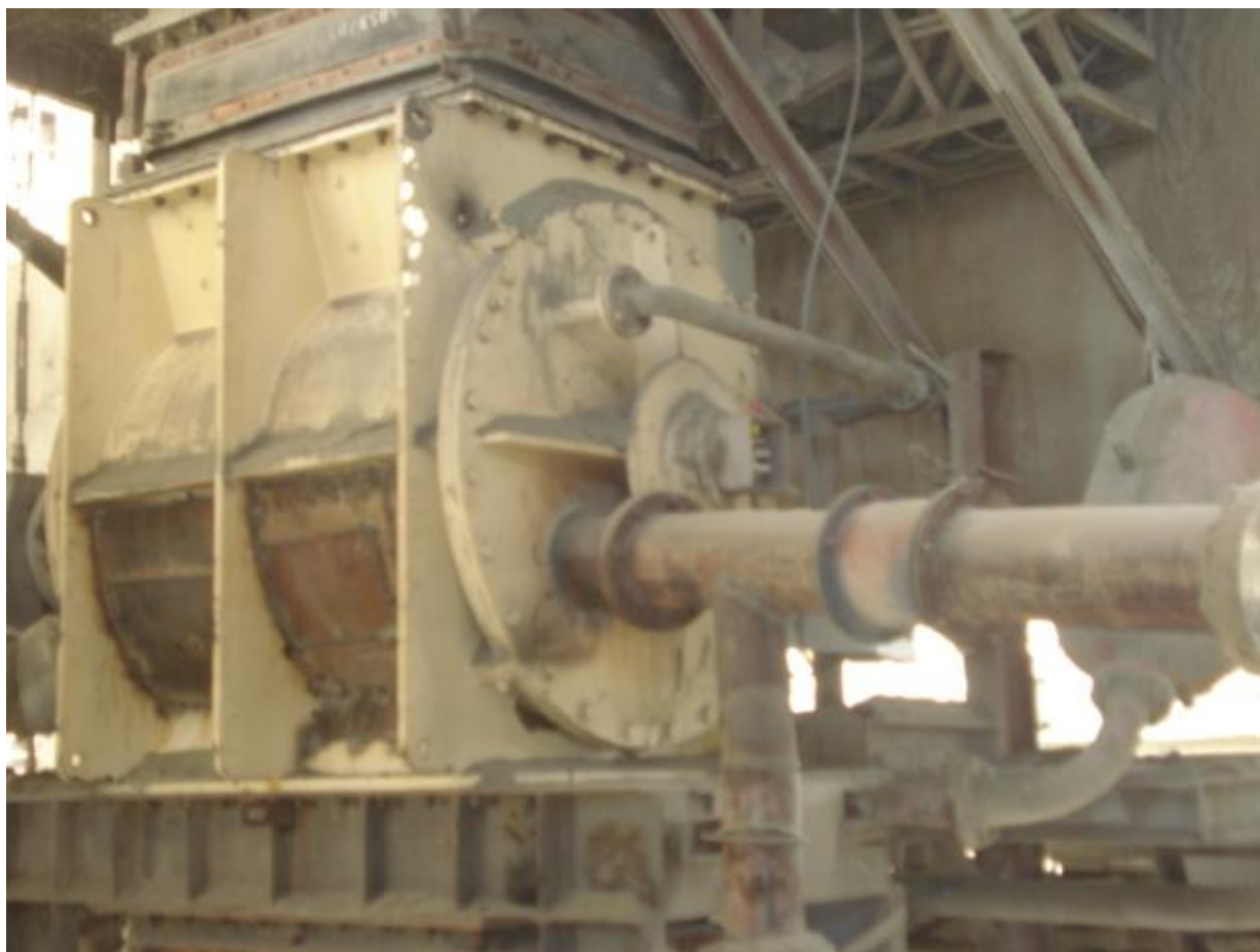
Star Feeder with HAG Pipe line connection
