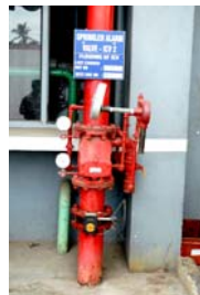
Sprinkler alarm valve
