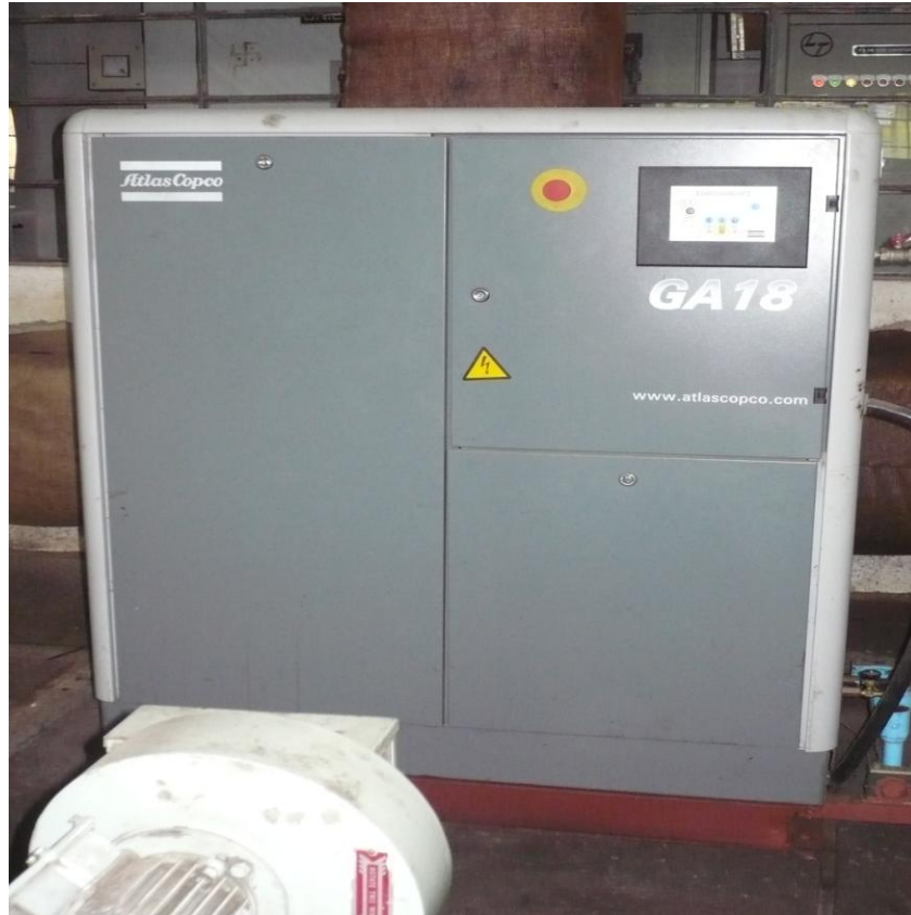
AIR COMPRESSOR PANEL 18.5 KW
