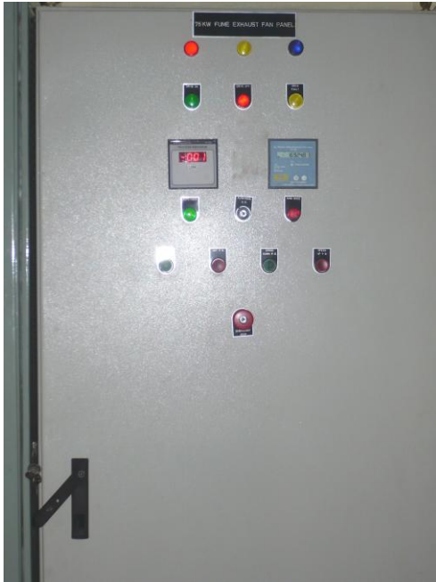
FUME EXHAUST SYSTEM : 75KW VFD
