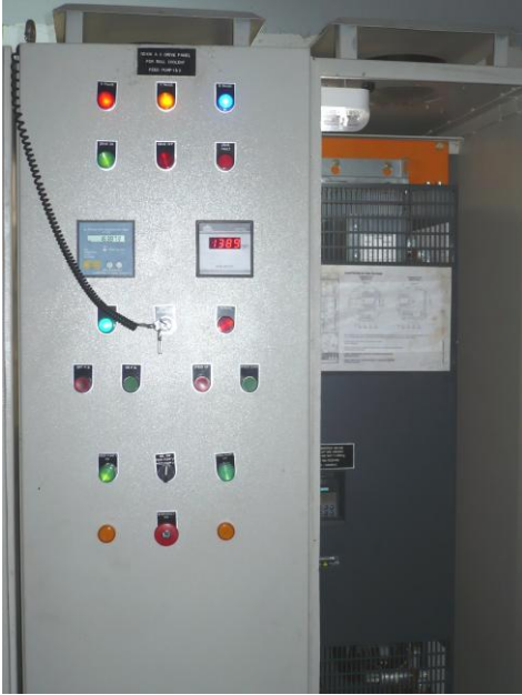
ROLL COOLENT FEED PUMP 110KW VFD
