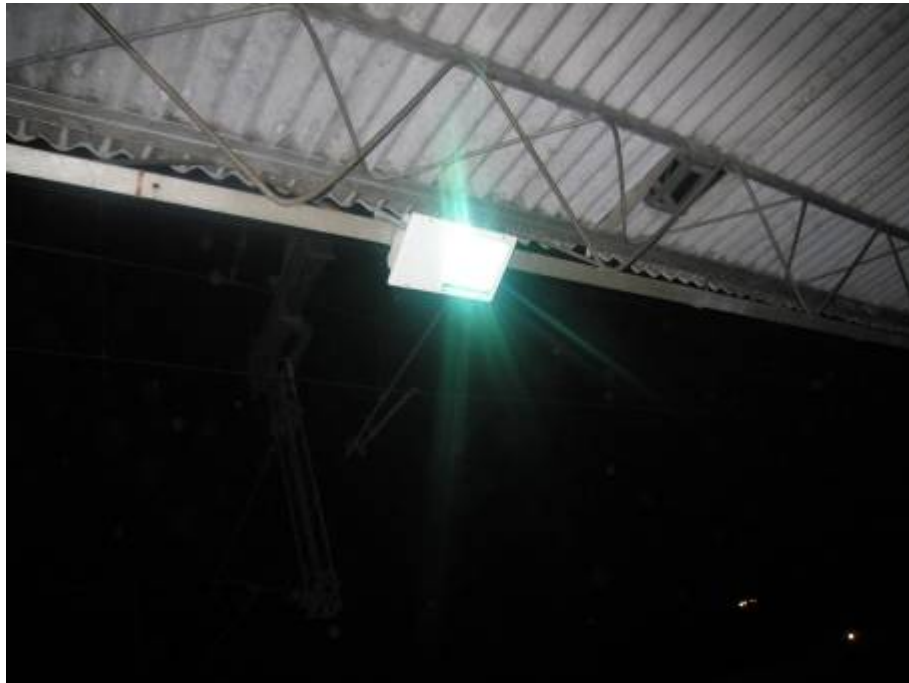
Use of 2x28 Watt Florescent Tube and 70 Watt Metal Halide Lamp
