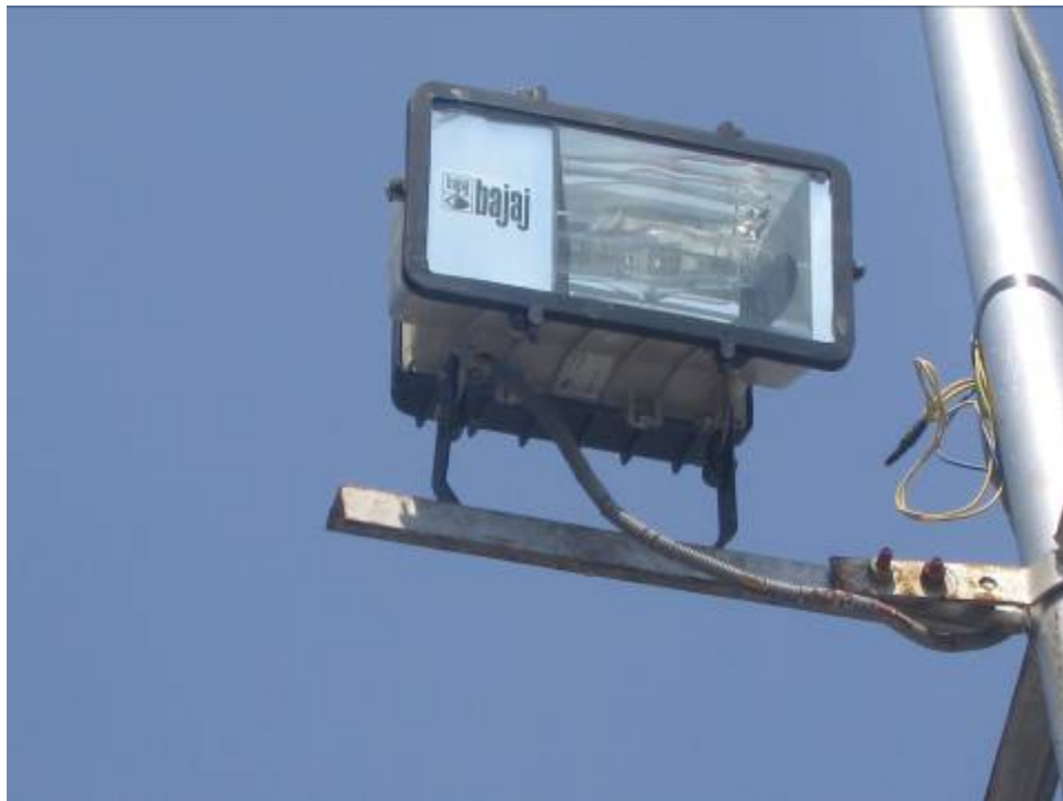
Use of 70 Watt Metal Halide Lamps in place of HPSV/HPMV Lamps
