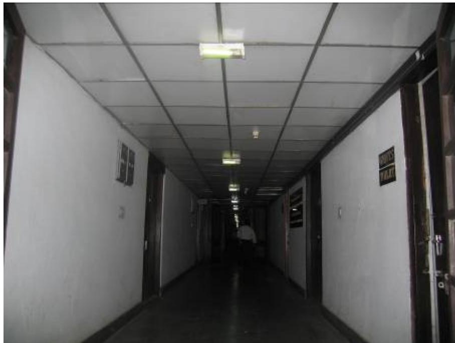
Compact Florescent Lamp (1x11 Watt) in place of 1x40 Watt Tube Light Fittings being used in Electrical Office, Baroda House
