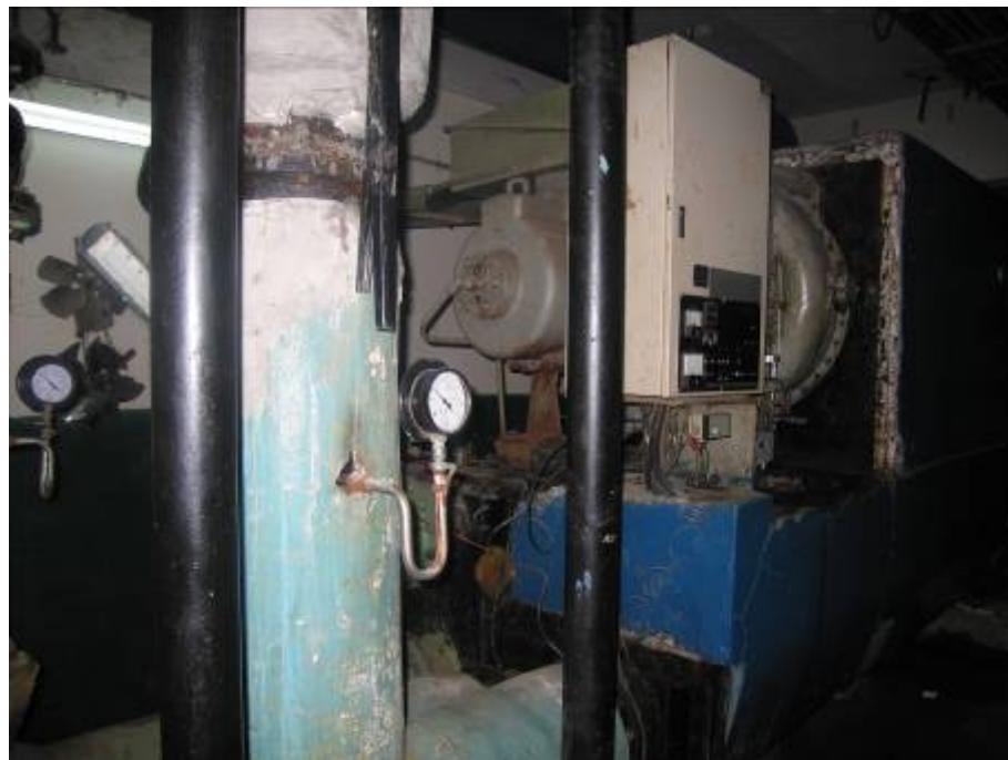
Use of LED Type Indication Lights and need based use of Central AC Plant in Baroda House Railway HQ Office
