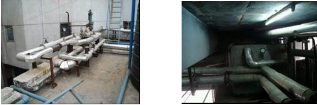
Figure 8: Hot Water Generators Installed in BHMRC
