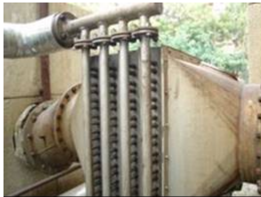
Figure 7: Economizer Installed in BHMRC
