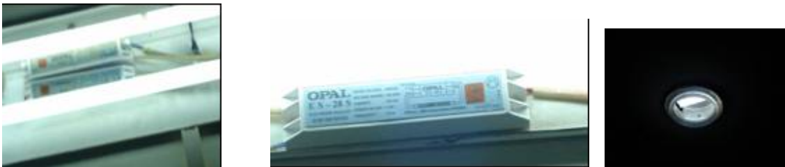
Figure 9: Lighting Retrofit Measures Implemented in BHMRC
