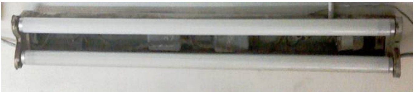
Old mirror optics fitting with copper ballast
