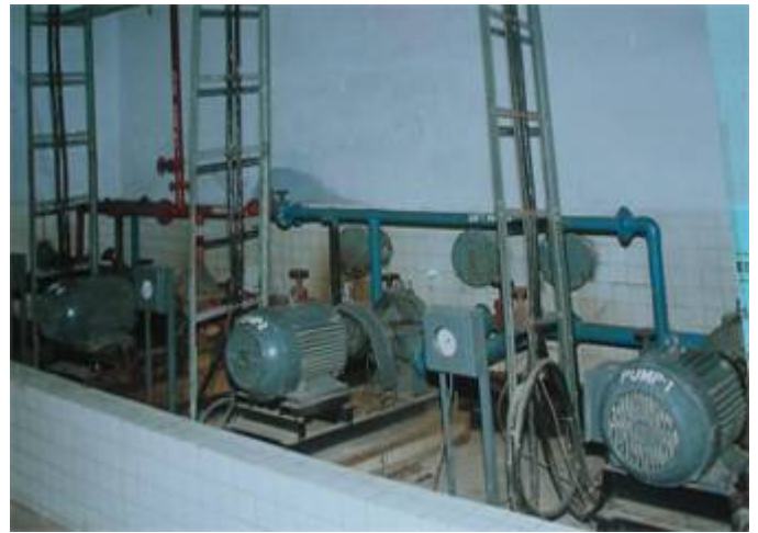
Old Energy inefficient pump sets
