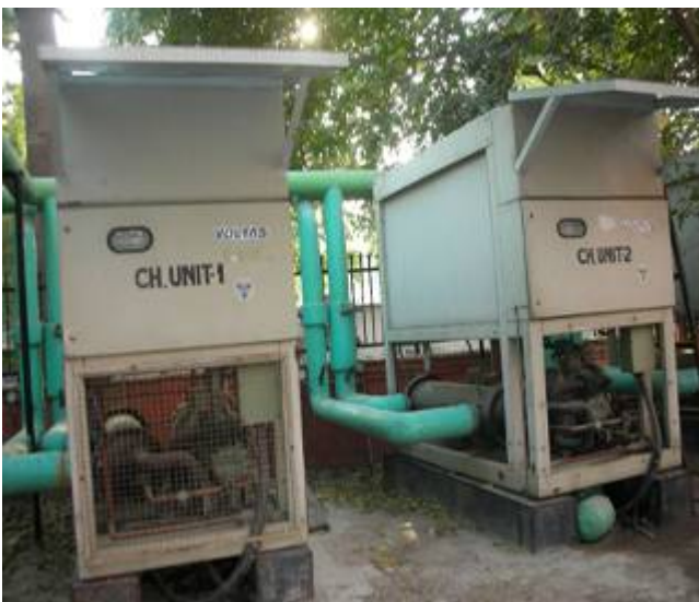
New Roof top Chiller
