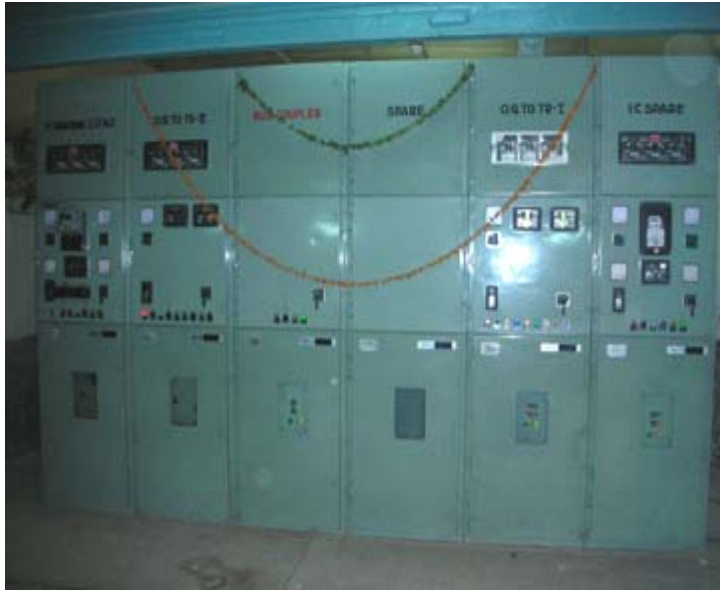
New Vacuum circuit breakers
