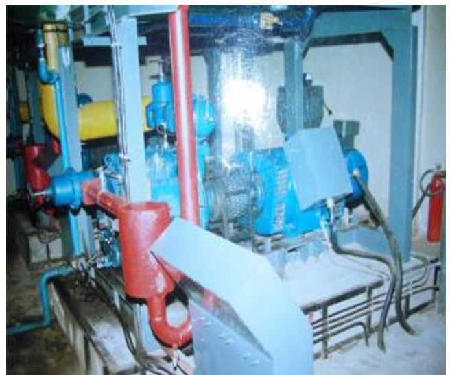
Old 2x64 TR Central AC Plant
