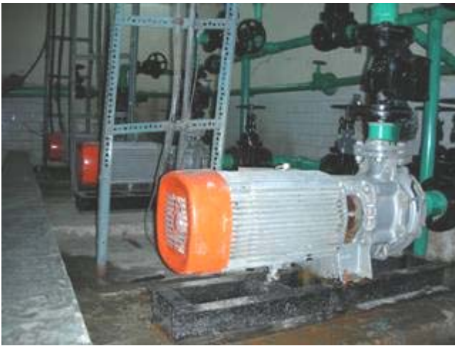
New Energy efficient pump sets
