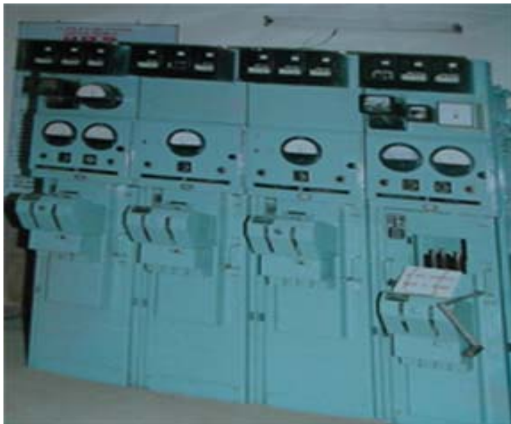
Old Oil Circuit breakers
