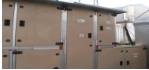
Heat Recovery Wheel
