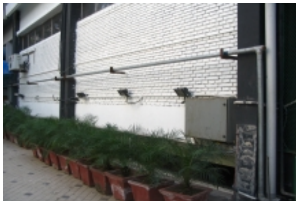
Soap free water pipeline going to the garden
