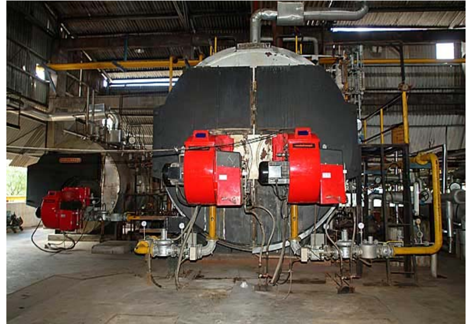
Gas Fired Burners Installed in Place of Conventional Low Efficiency Furnace Oil Burners
