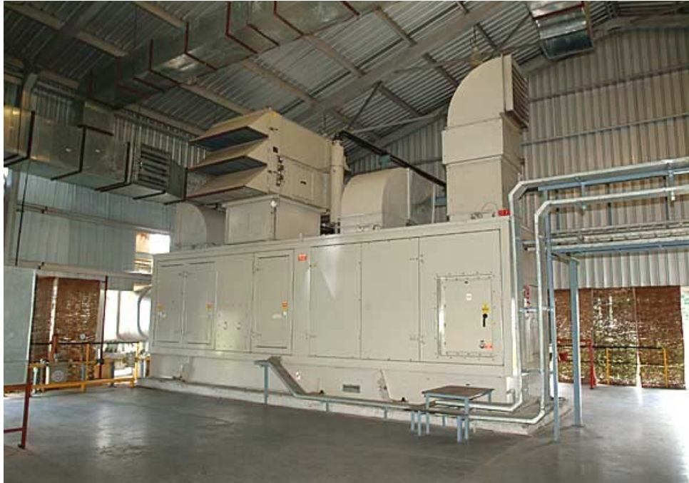
Low NoX Natural Gas based Engine & Turbine Installed for Co-Generation
