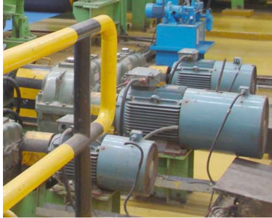
AC motors in Colour Coating Line 1
