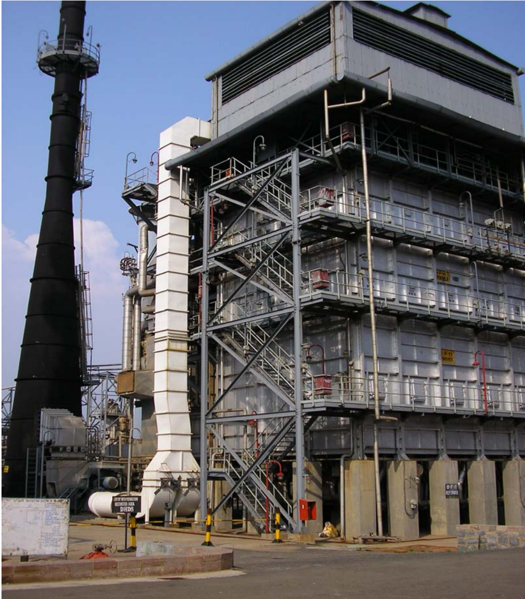
Hydrogen Unit Reformer: (provided with Air Pre heater and steam drum which recovers heat from flue gases for air pre-heating and generation of High Pressure Steam.)
