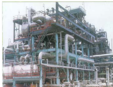
Standby Sulphur Recovery Unit
