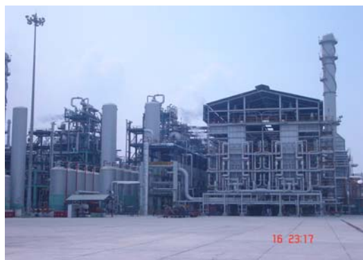
New Hydrogen Generation Unit
