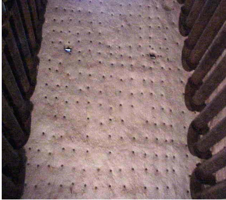
Ceramic Insulation Inside Furnace
