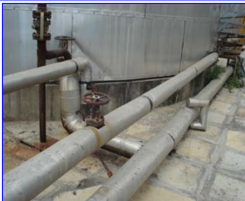
Steam supply ON.
