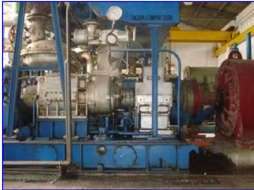
HT screw compressor capacity 5000NM 3 /Hr
