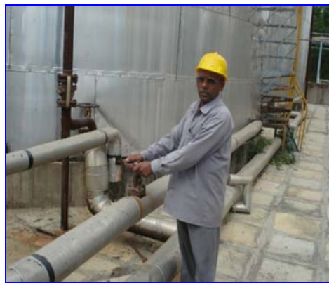
Steam supply to FO tank coil & jacketed line stopped.
