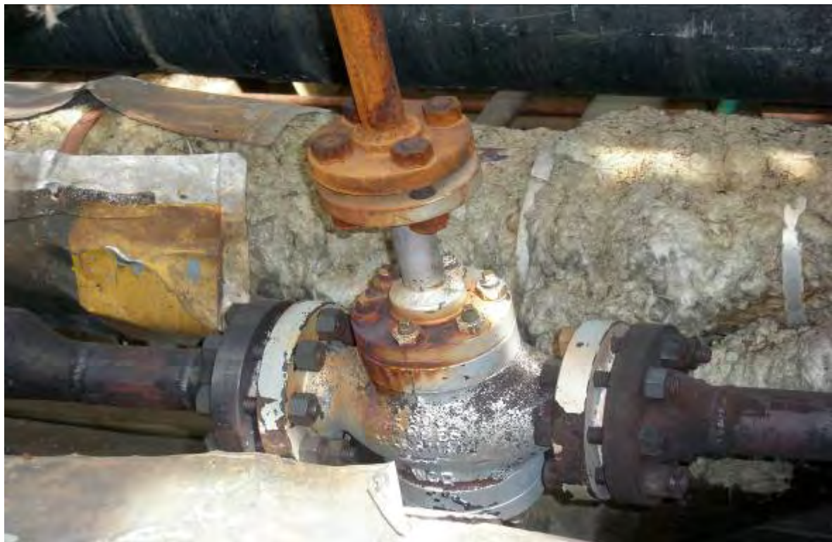
( De-Superheater Condensate Spray nozzle installed in Polypropylene Co-polymer plant )
