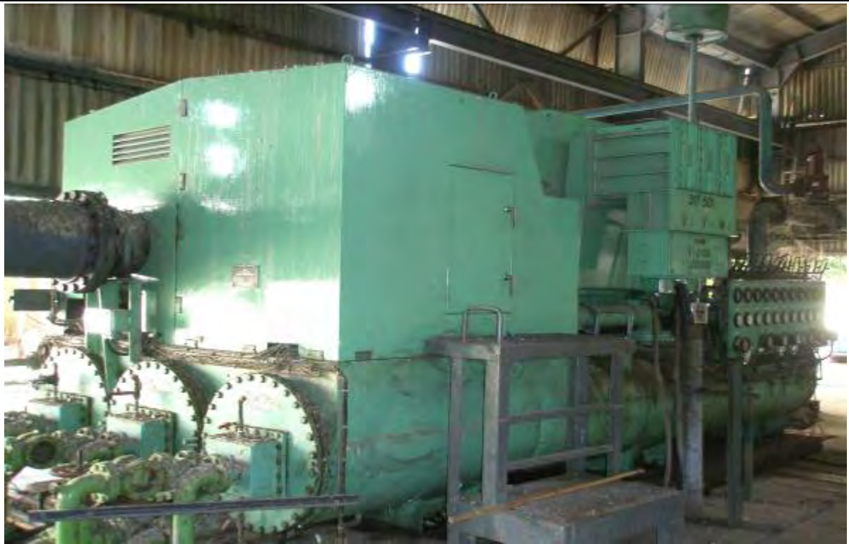
(Photograph showing other side view of Mitsubishi Air Compressor for which overhaul job was carried out for improving Energy Efficiency and performance)
