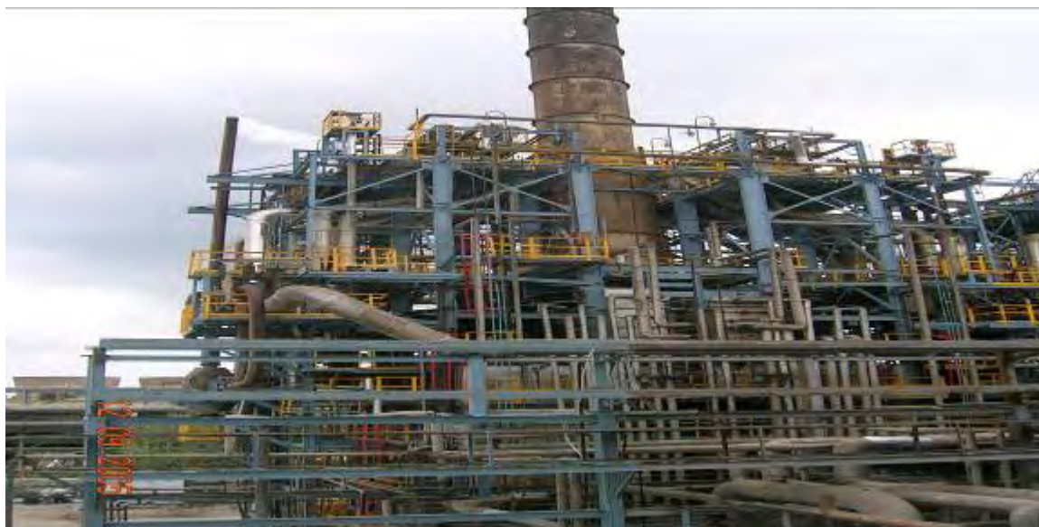
(Photograph of a section of SRT Heaters before modification)
