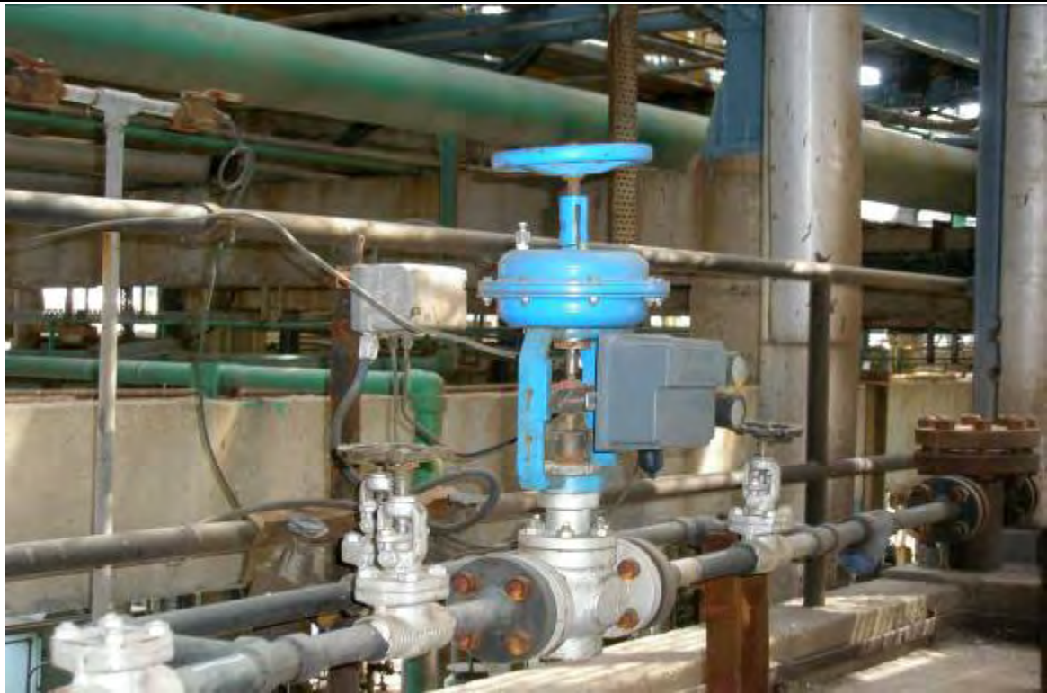
( De-Superheater Control valve installed in Polypropylene Co-polymer plant )
