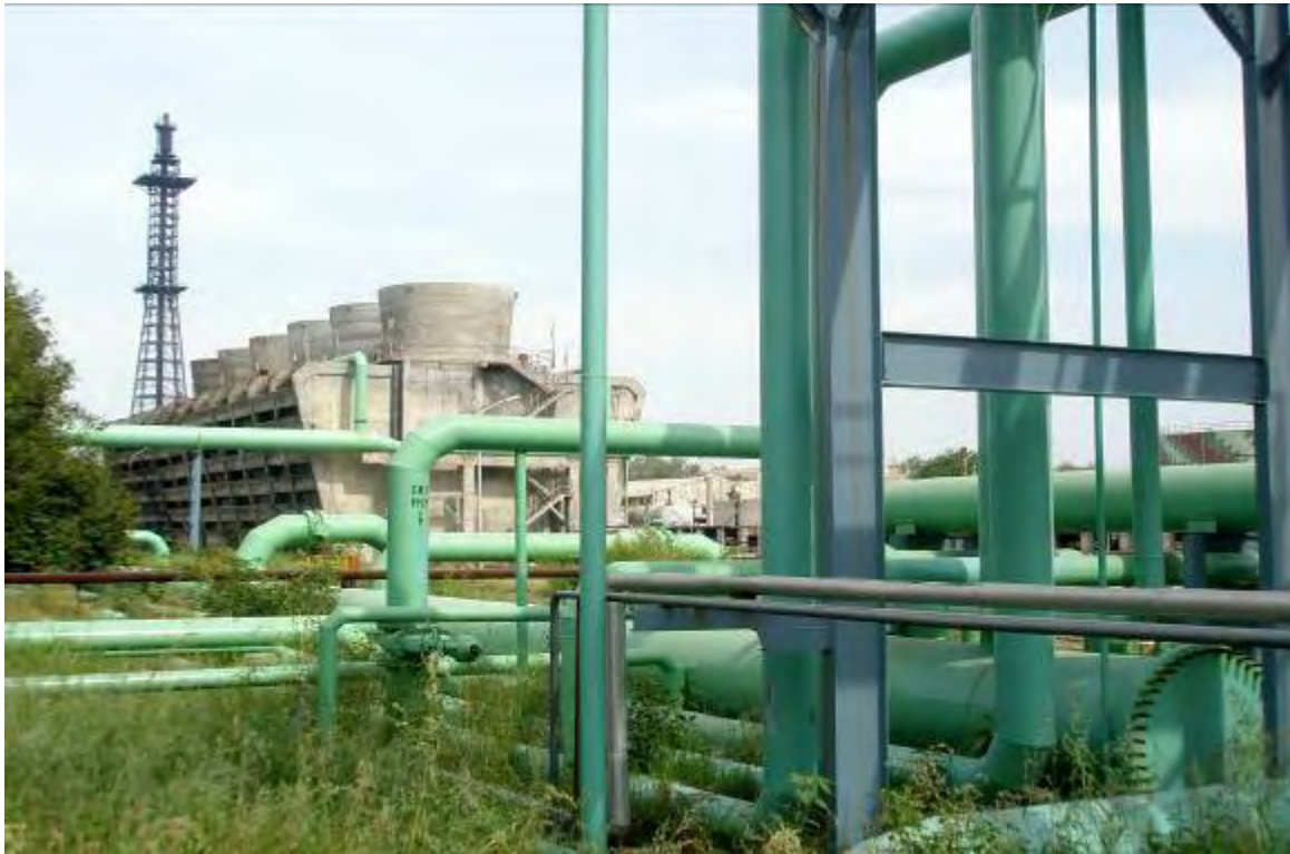
( Photograph showing partial header network of the CW system of Utilities plant )
