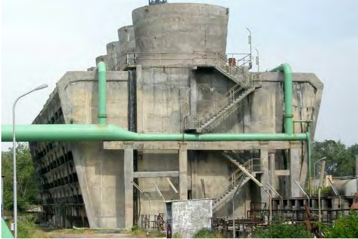
( Photograph showing Cooling Tower of Utilities plant which was taken up for Energy Audit study of CW network system )
