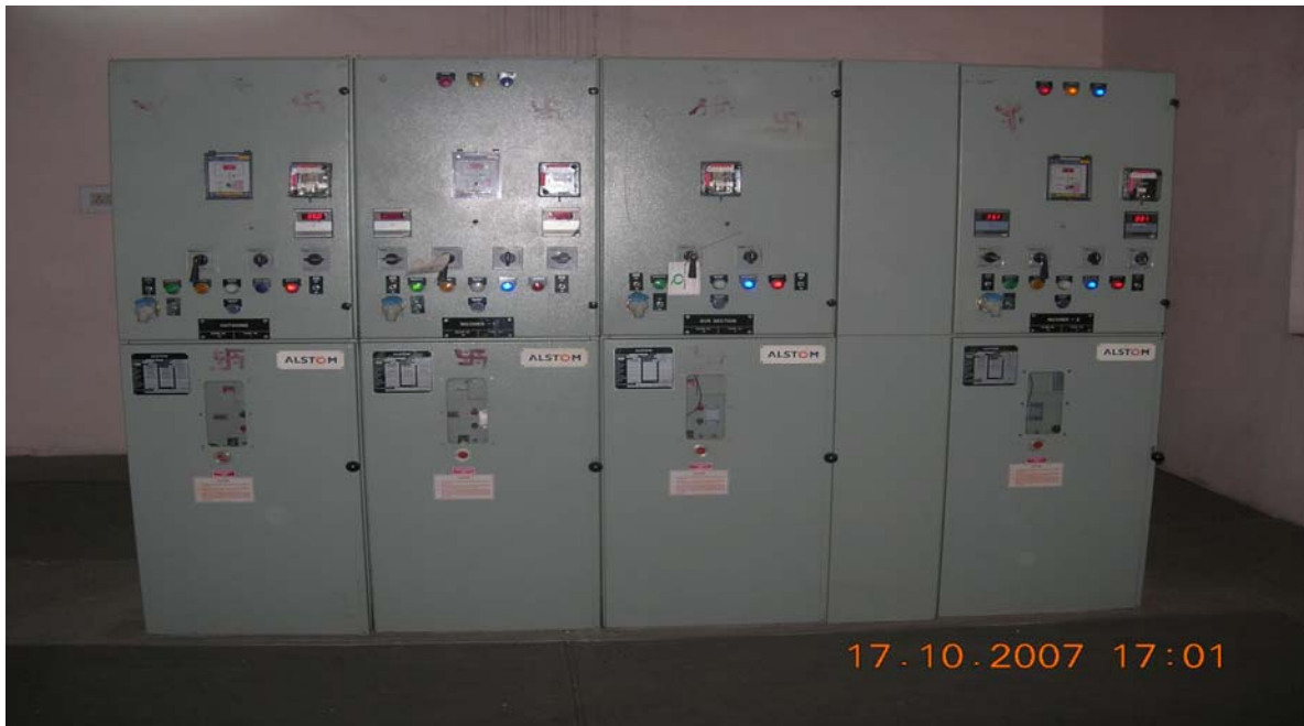
11 KV MOTORIZED PANEL AT 33 KV SUB STATION, BALAGHAT MINE, MOIL
