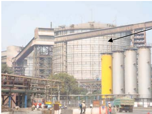
Photograph showing the new LD gas Holder
