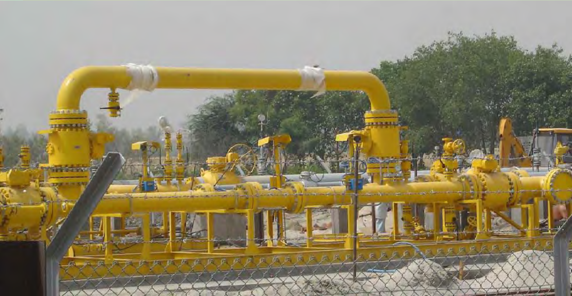
RLNG METERING SKID AT GAIL SITE
