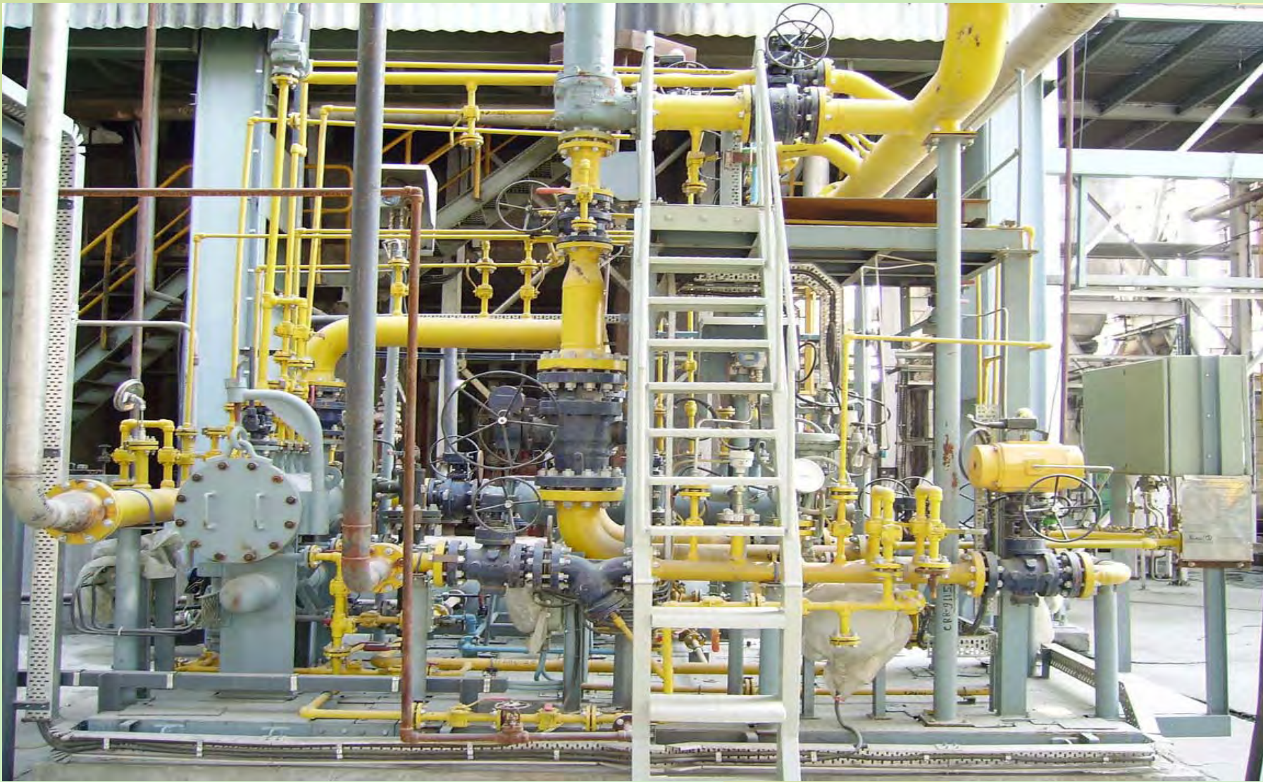
R-LNG Control Station in Amm.- I Plant
