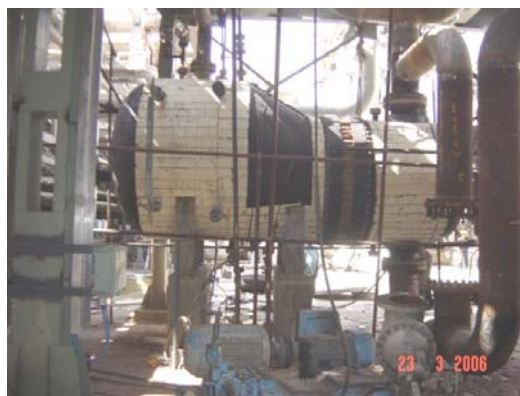
New Make-up Gas Chiller
