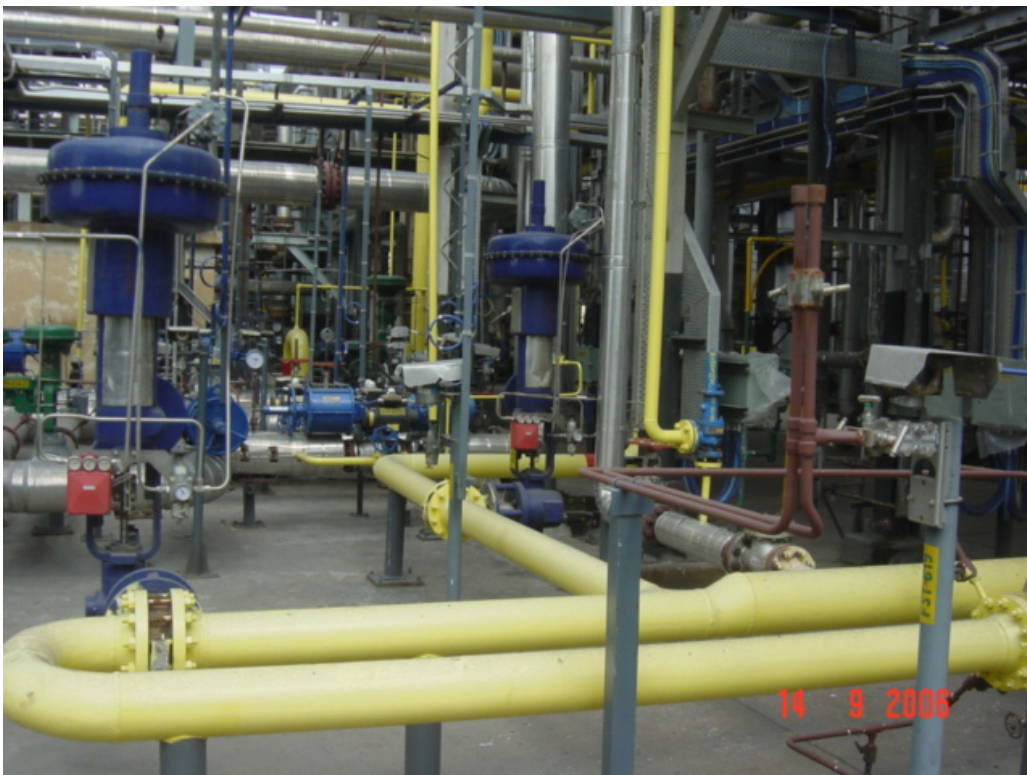
RLNG FUEL LET DOWN STATION
