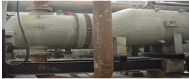
Final Gas Chiller
