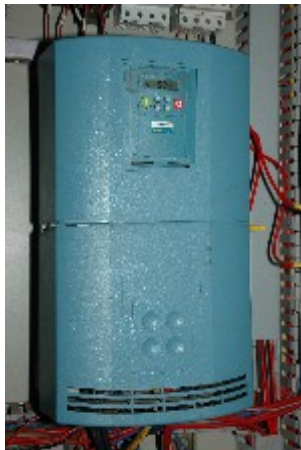
VFD for DEO pump (803)
