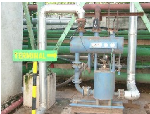
Condensate recovered from terminal section
