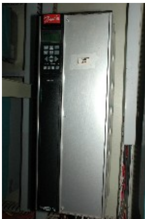
VFD for fatty acid pump (804)
