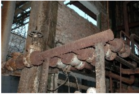
Flash steam header with NRV arrangement
